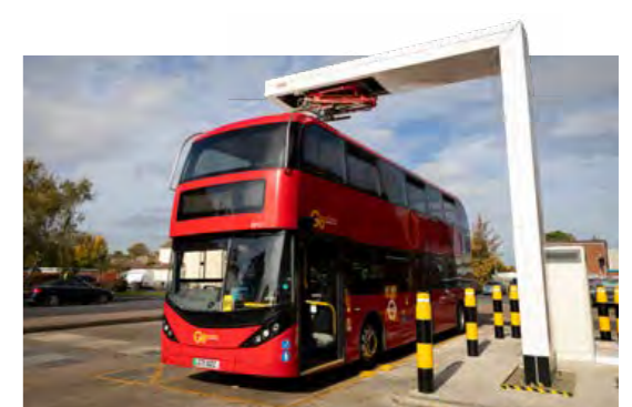
October 2022 Rapid, wireless bus charging technology is introduced as part of our journey to zero-emission carbon
